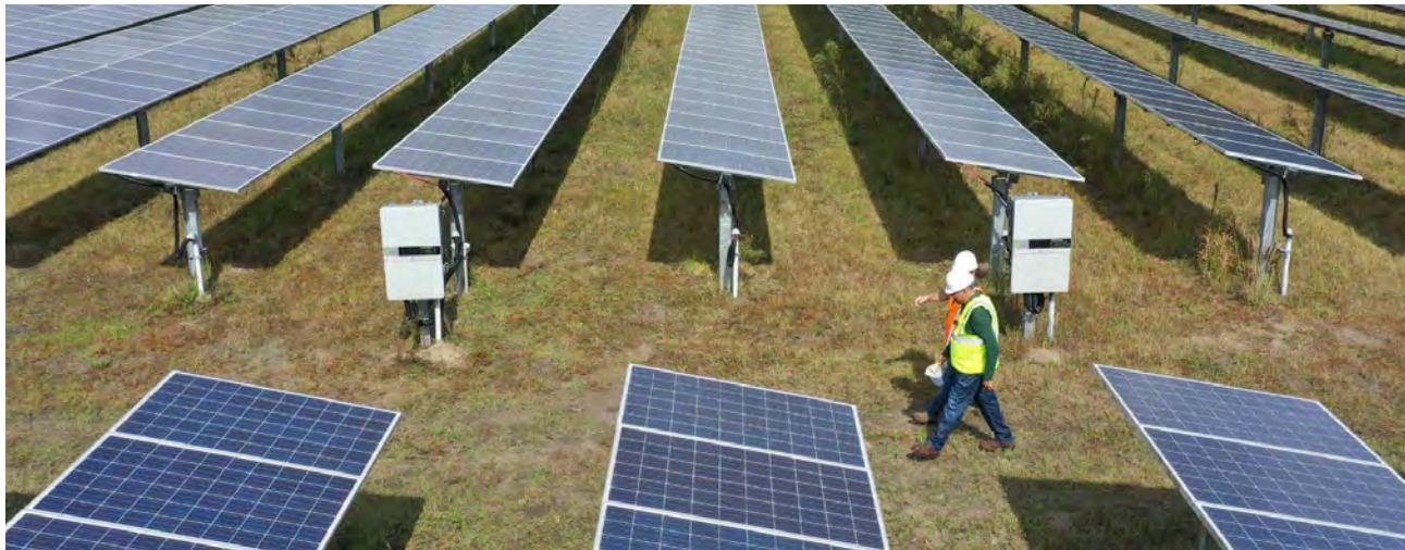
Blair Road Solar, Jacksonville, FL
